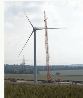
4. Once final checks are completed, the turbine is ready to generate renewable energy
